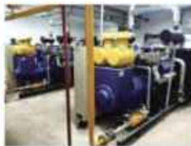
菲律宾某污水处理厂电站项目 A sewage treatment plant power station project in the philippines
